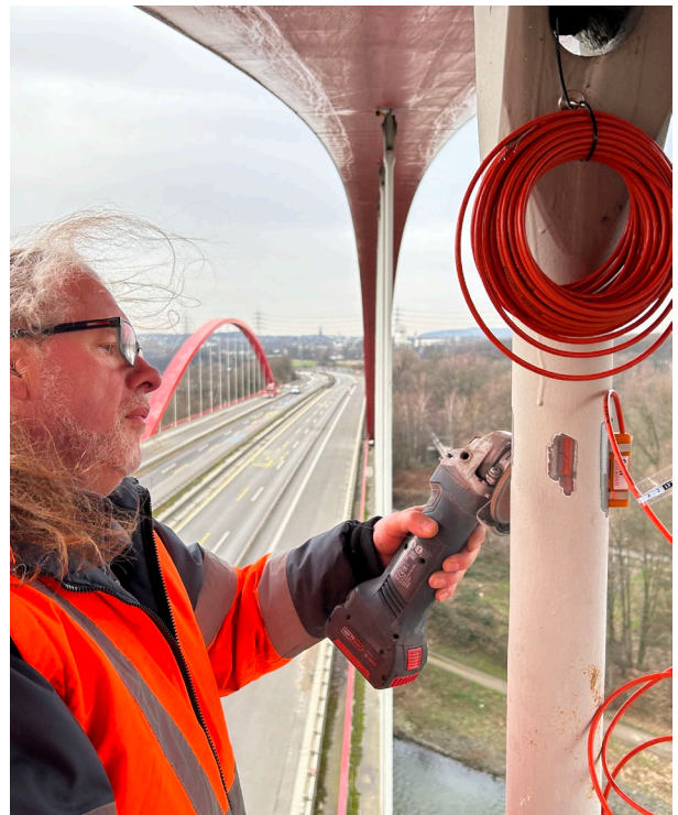
Installation of sensors on the A42 motorway bridge over the Rhine-Herne Canal (Germany)
